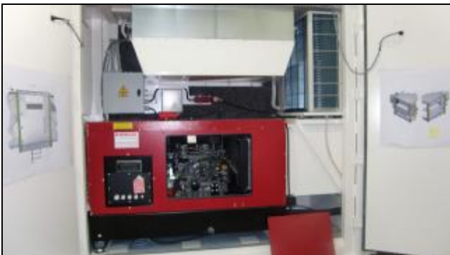
Technical room with power generator
